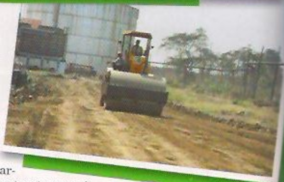
The application of these stabilisers involves the standard procedure of road construction.
